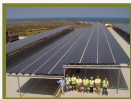
250 kW Photovoltaic Array
